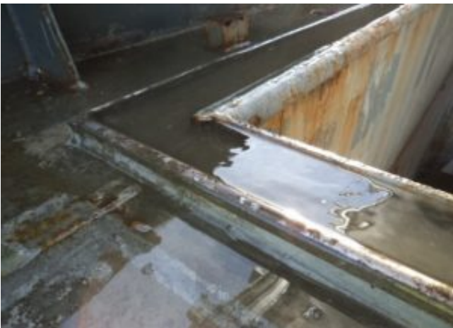
Figure 3: Overflowing drainage channels
